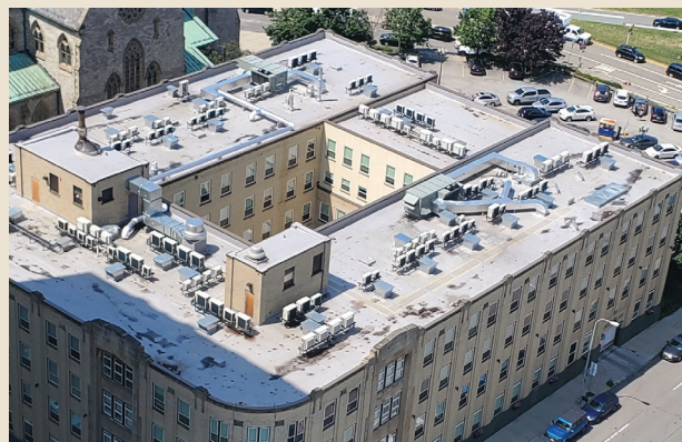
Commercial air source mini-split heat pumps at the Police Apartments in Buffalo, NY.
