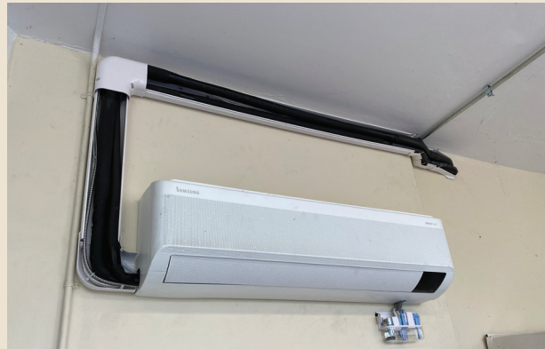
VRF at the Erie County Board of Elections building.
