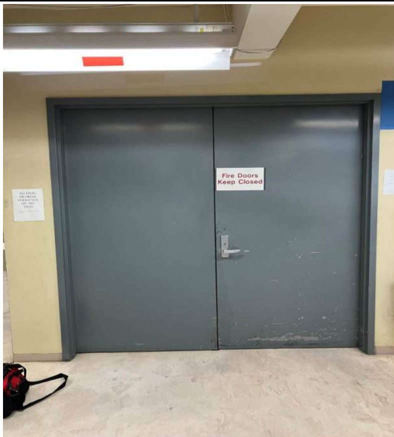
Photo 5: Photograph of the elevator lobby doors on floor Tier A. Grey metal door slabs and frames were found to be coated in lead-based paint on the Tier Floors.
