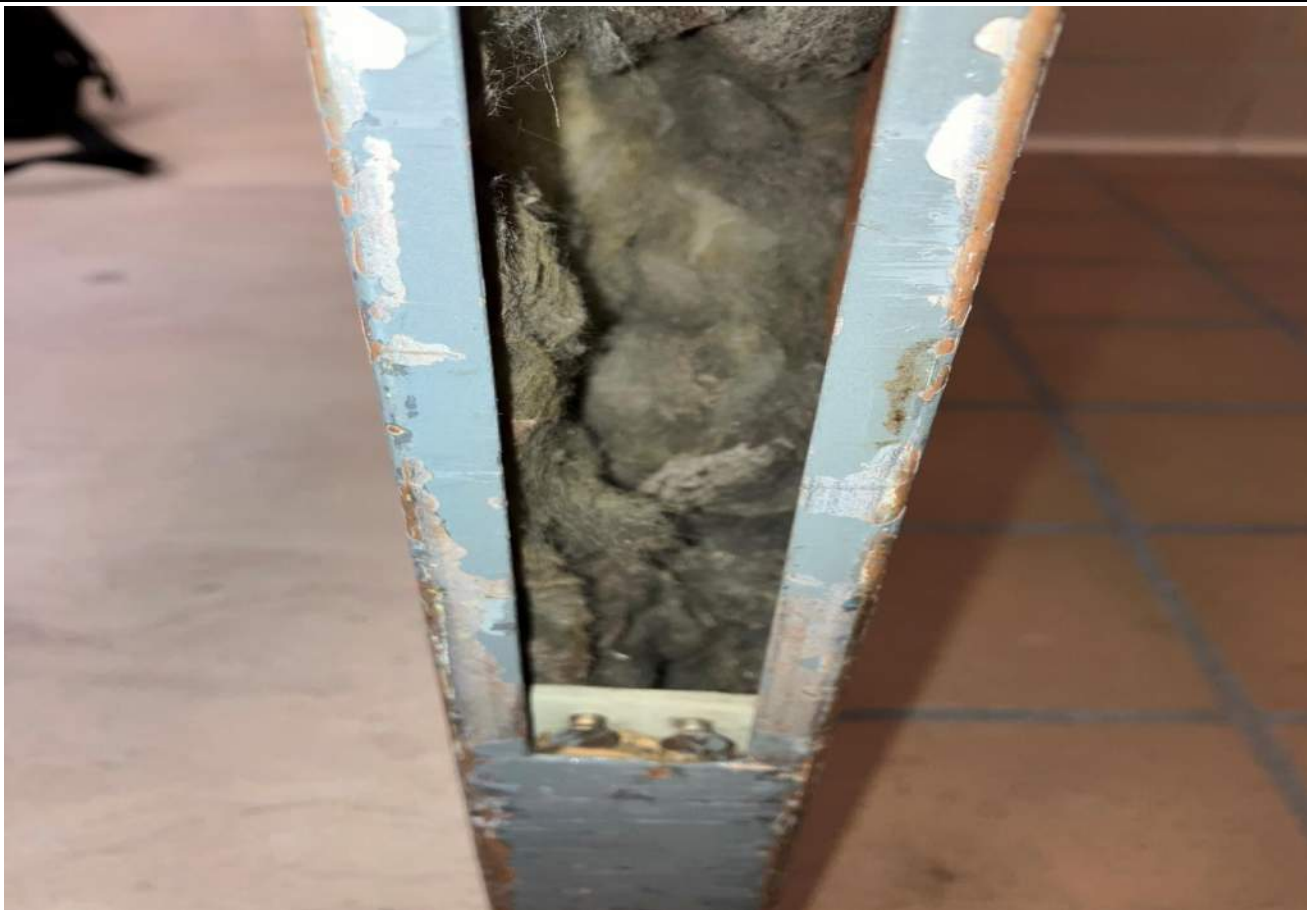
Photo 6: Photograph of the non-suspect fiberglass insulation found in fire doors on floors Tier A and Tier B.
