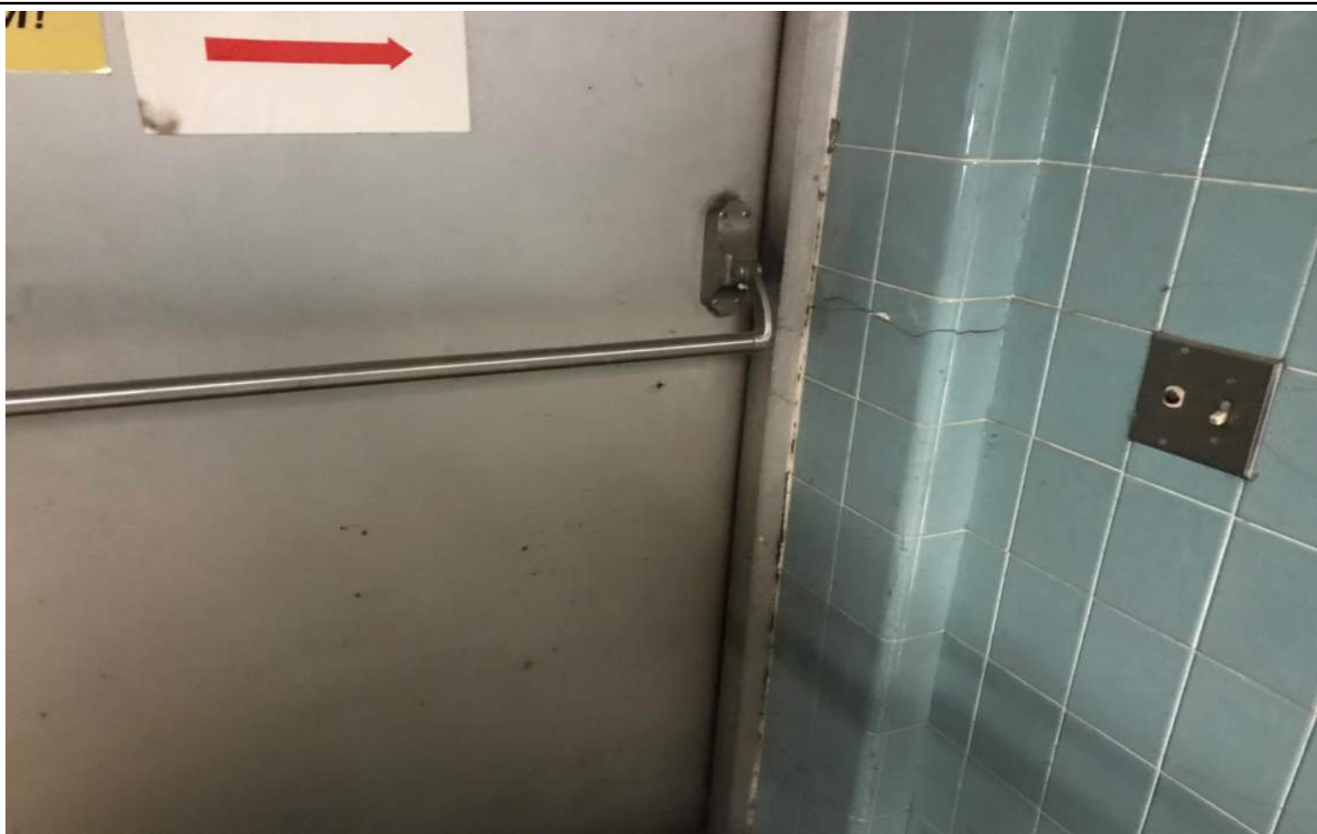
Photo 3: Photograph of the ceramic wall tile in East Penthouse stairwell. The grout and mudset were determine to be non-ACM.
