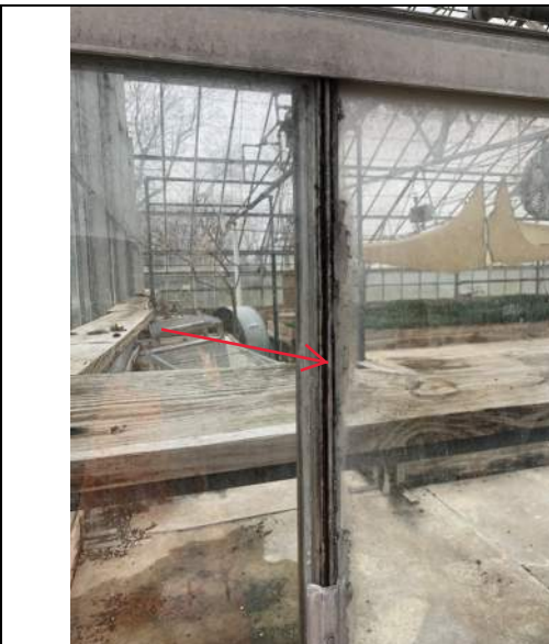
Caulking for Glass, Under Metal Trim - Asbestos Containing Material
