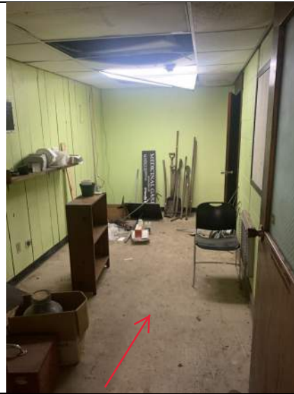
12x12" Floor Tile, Gray – Asbestos Containing Material
