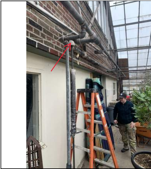
Mudded Joint Fitting associated with 504 - Asbestos Containing Material
