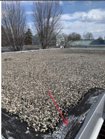
Silver Seal, Silver - Asbestos Containing Material
