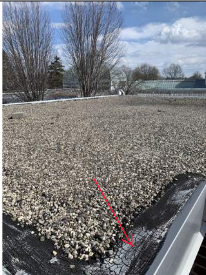
Silver Seal, Silver - Asbestos Containing Material
