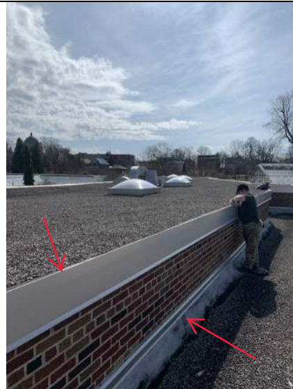
Silver Seal, Silver - Asbestos Containing Material
