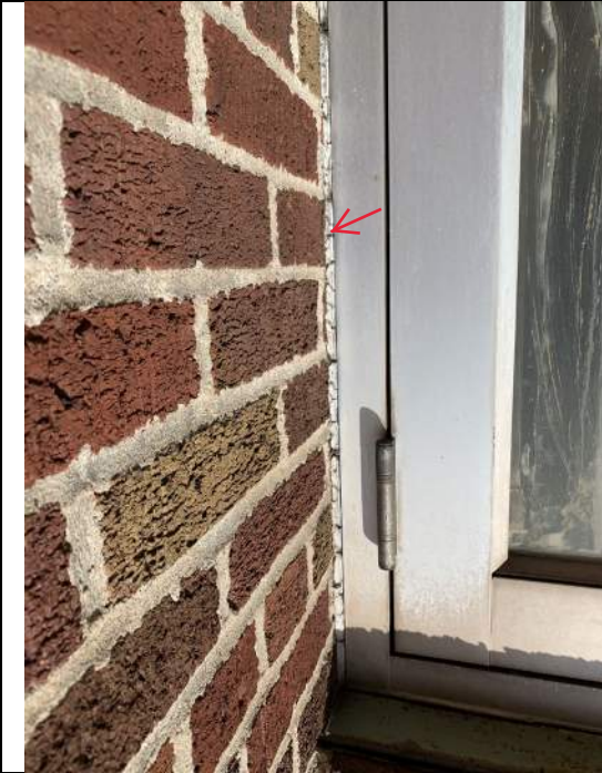
Caulk around Double doors, White – Asbestos Containing Material
