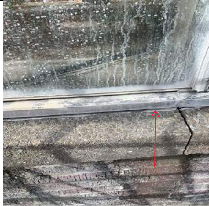
Caulk, Gray, Greenhouse 1 and 2, between Glass and Concrete –Asbestos Containing Material
