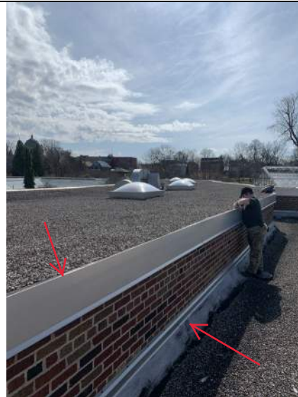
Silver Seal, Silver - Asbestos Containing Material
