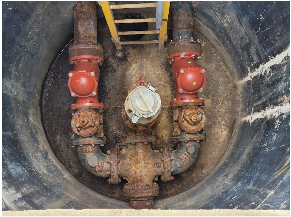
Figure 2-12: EHPS Valve Vault
