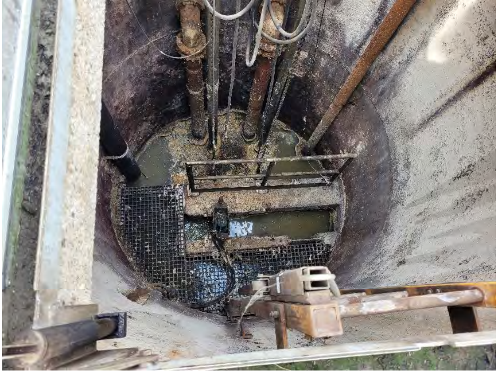
Figure 2-11: EHPS Wet Well
