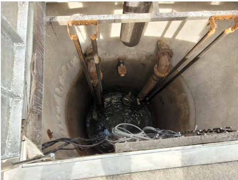
Figure 2-14: BPS Wet Well
