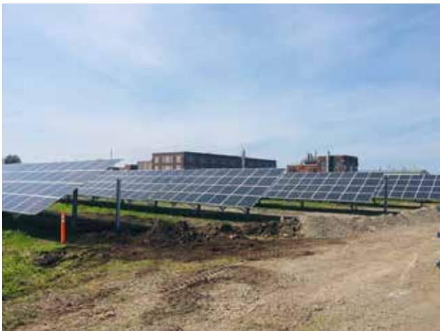
New Solar Array on Woodward Avenue
