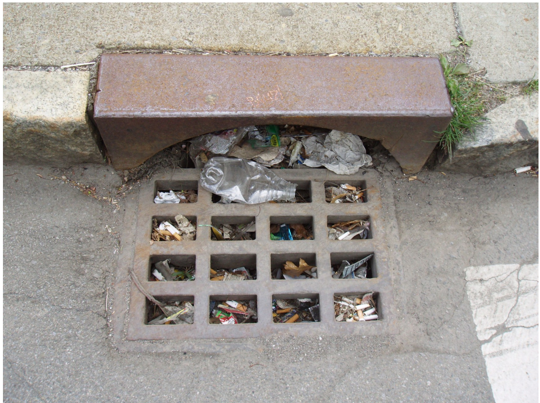
Clogged Storm Drain
