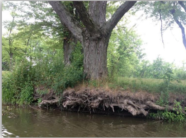
Ellicott Creek Erosion (Tonawanda, NY) Courtesy of Buffalo Niagara Riverkeeper
