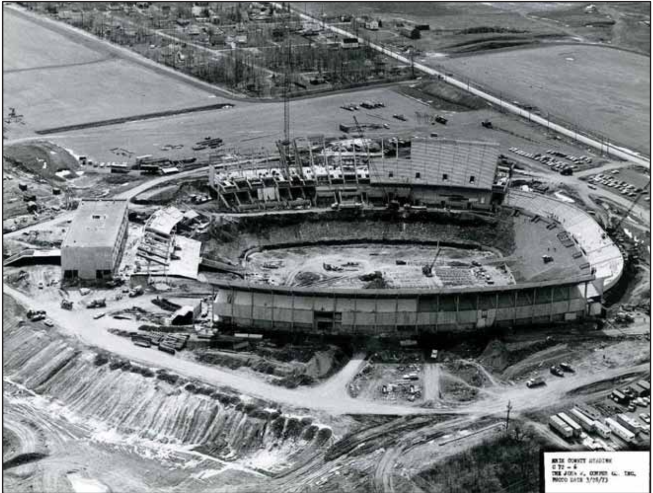
Figure 2.5. An aerial view of the stadium construction on March 28, 1973, facing southwest ( Courtesy of the Buffalo Bills ).
