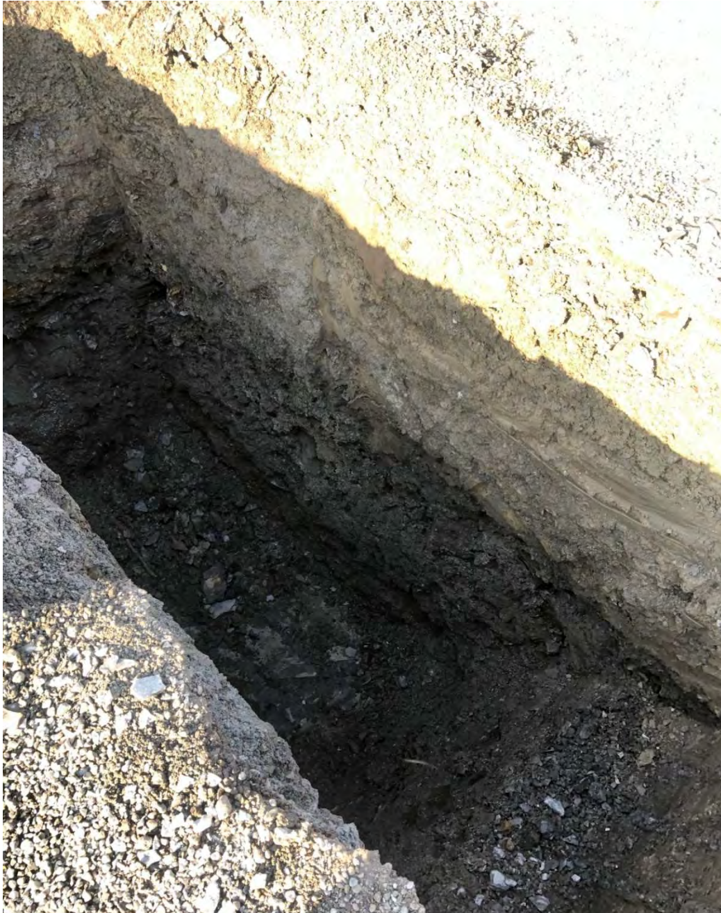
TEST PIT TP-1-22. Bottom of test pit at 11.3 feet deep. Transition from overburden to weathered rock at approximately 10.0 feet, and transition to competent rock at approximately 10.7 feet.
