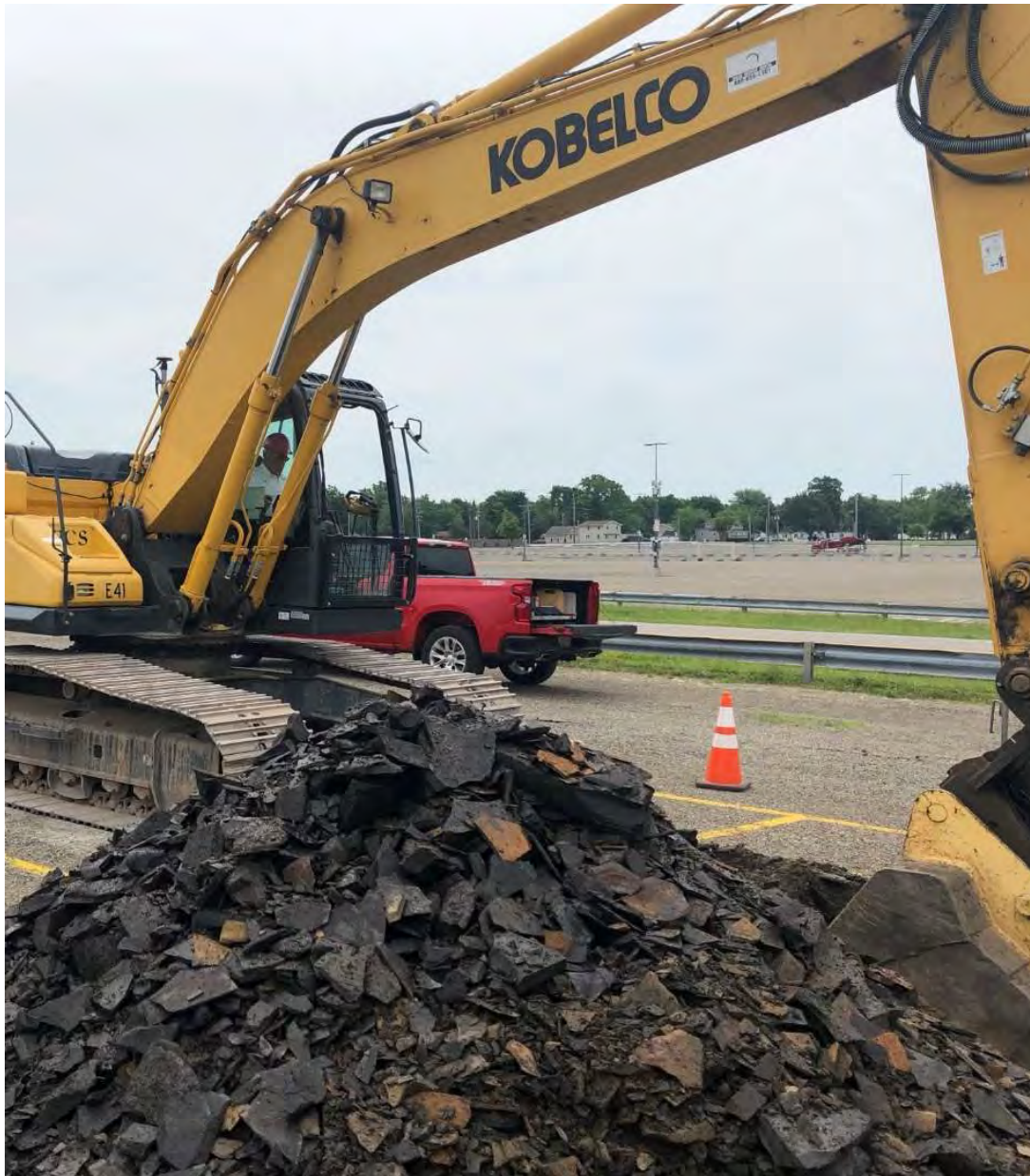
TEST PIT TP-2-22. Excavated weathered rock with excavator (Kobelco SK210 LC) for scale.
