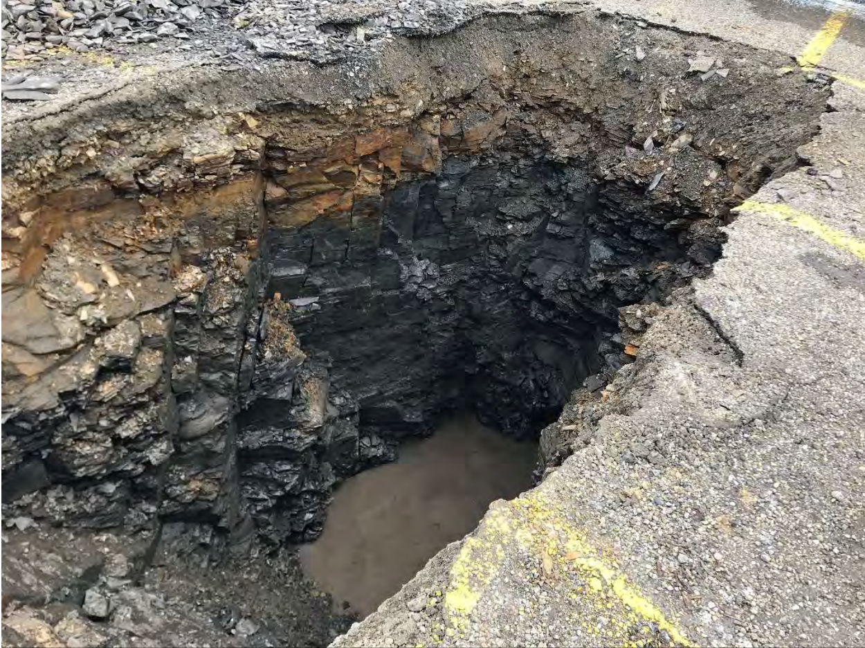
TEST PIT TP-2-22. Water began infiltrating the excavation at a depth of approximately 10.0 feet.
