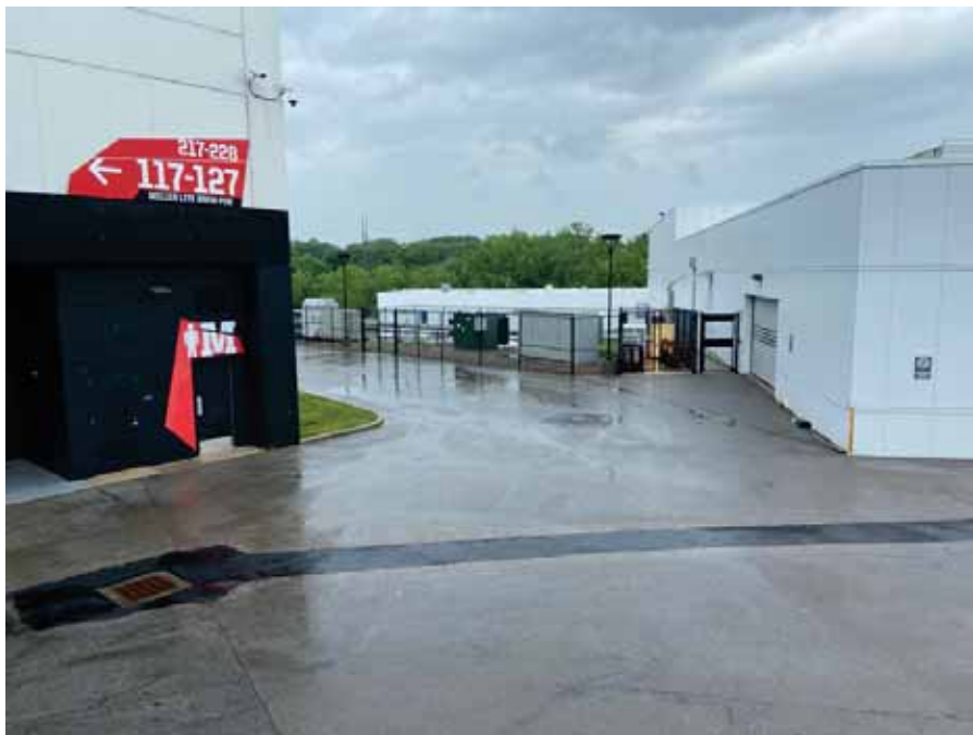
Photo 50 : Pad-mounted transformers located on the southeastern exterior of Building One
