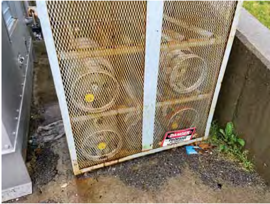
Photo 59 : Propane located east of Building One
