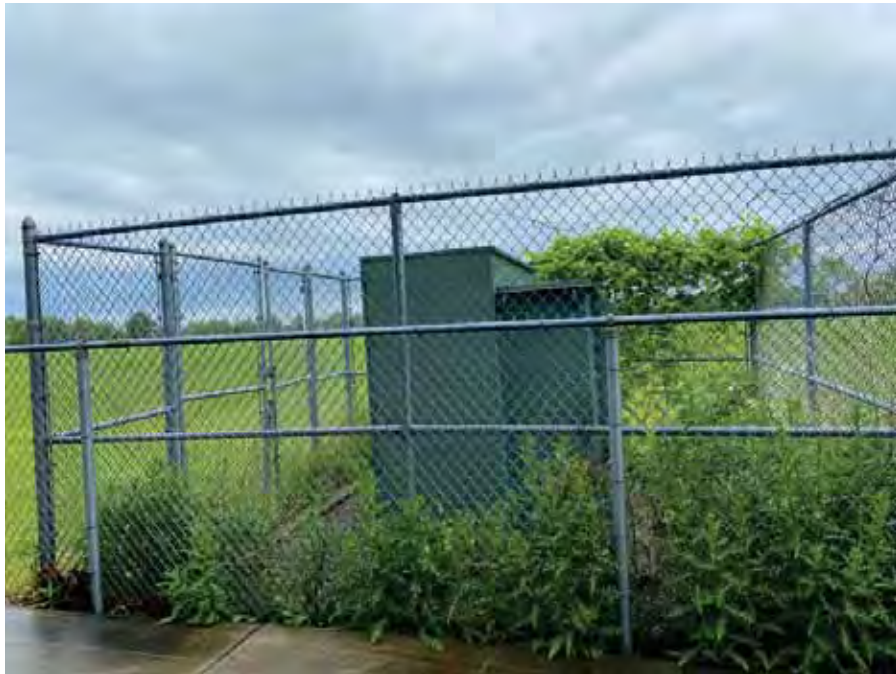
Photo 136 : Pad-mounted transformer located north of bleachers on ECC campus in Area Two
