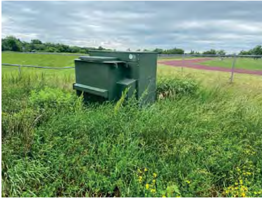
Photo 139 : Pad mounted transformer located on Area Two
