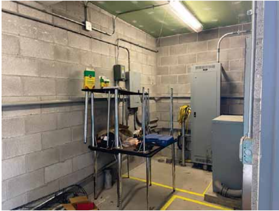
Photo 135 : Pad-mounted transformer in storage building underneath bleachers in Area Two
