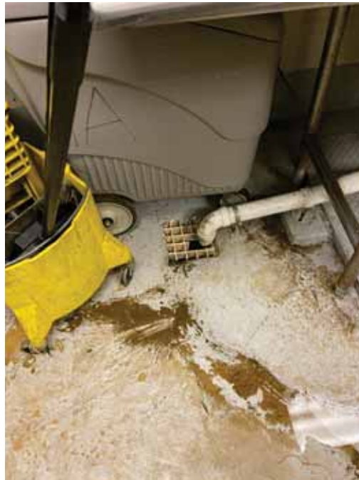
Photo 42 : Typical drain located within janitor closet
