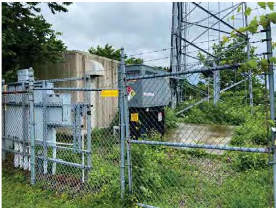
Photo 120 : Diesel generator located next to cell phone tower
