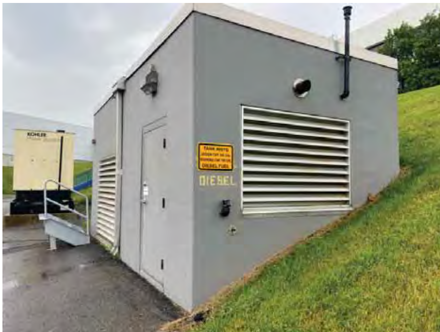
Photo 56 : 200-gallon diesel AST for generator
