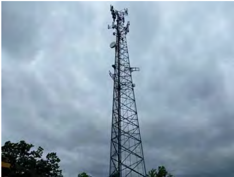
Photo 119 : Cell phone tower located north of Building Eight
