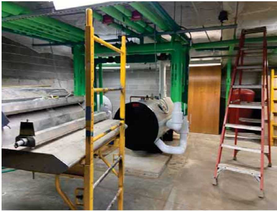
Photo 35 : Typical boiler room in Building One
