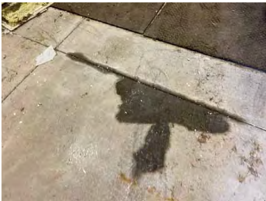
Photo 134 : Staining observed in shed underneath the bleachers in Area Two
