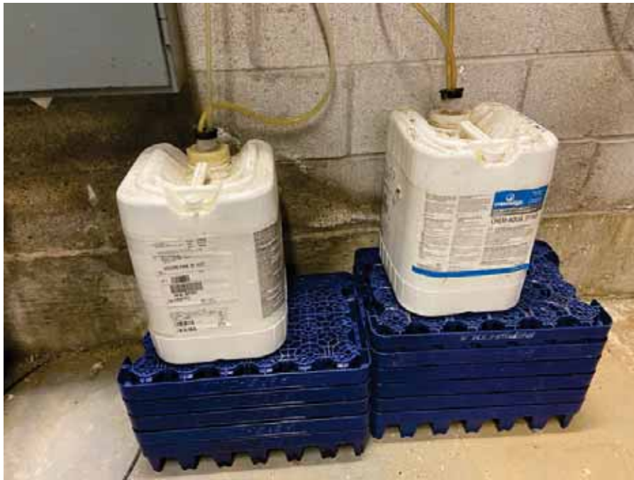
Photo 47 : Typical water softeners in Building One
