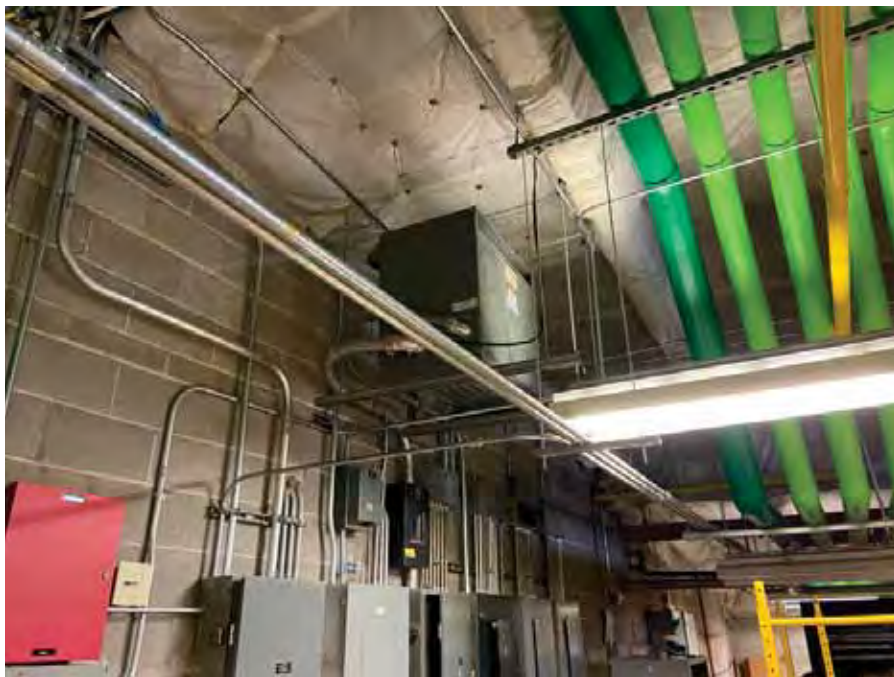
Photo 36 : Typical transformer in Boiler Room in Club Areas in Building One
