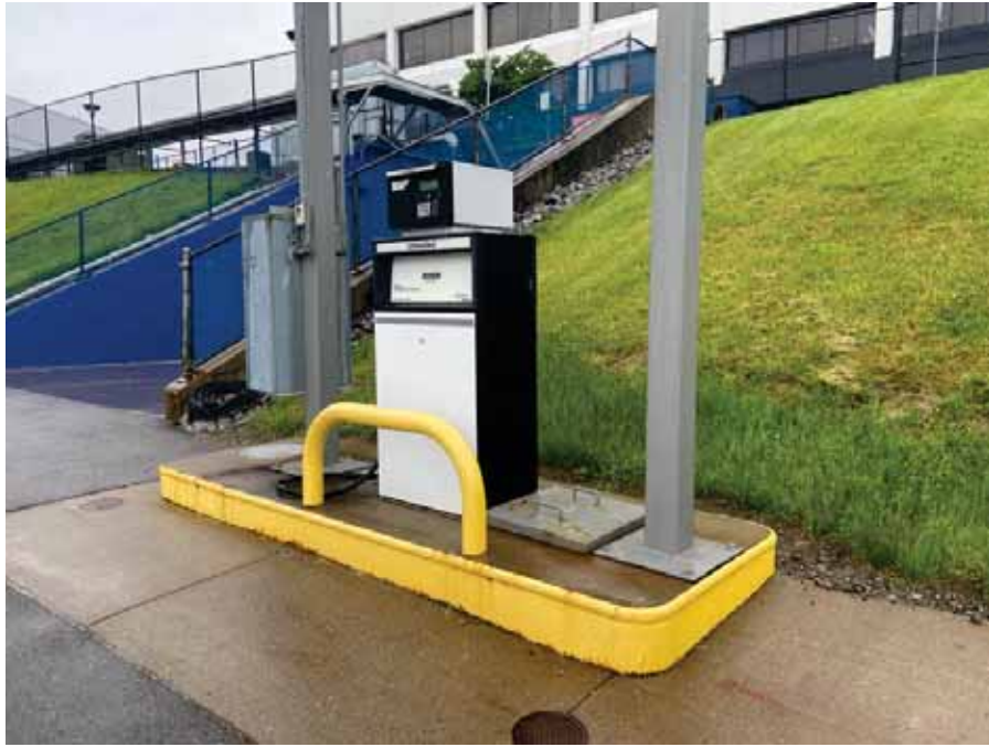
Photo 53 : Dispenser for diesel fuel
