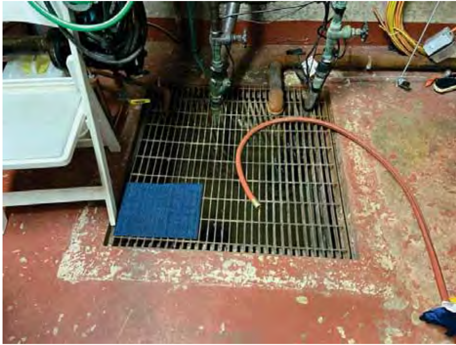
Photo 41 : Sump Pump located within Building One
