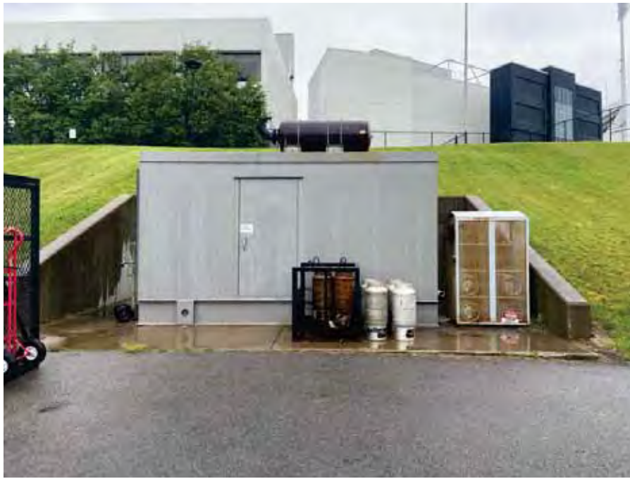
Photo 55 : Diesel Generator and propane
