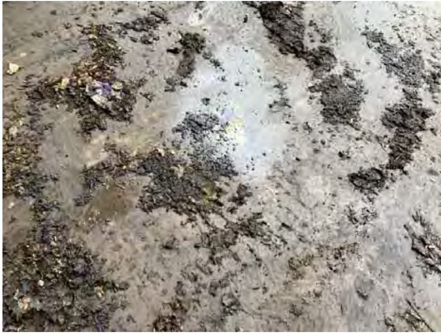
Photo 115 : Minor oil staining observed in Building Eight
