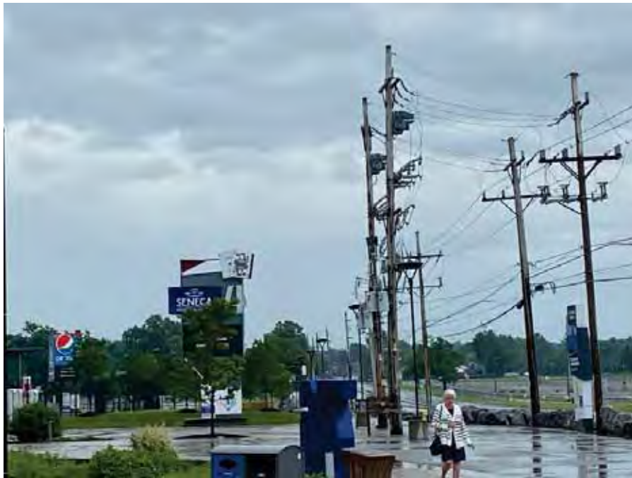
Photo 77 : Pole-mounted transformers located south of Building Three
