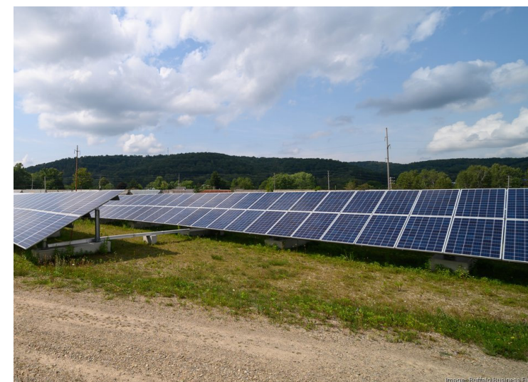
Solar Panels in Olean, NY By: Joed Viera
