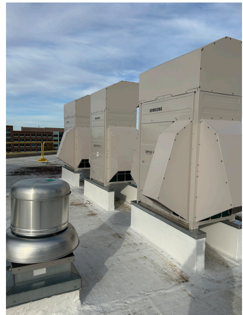
- Heat Pumps on the Erie County Board of Election Building
