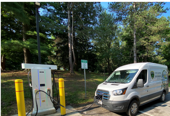
- Erie County EV being charged at Level 3 Charger at Akron Falls Park
