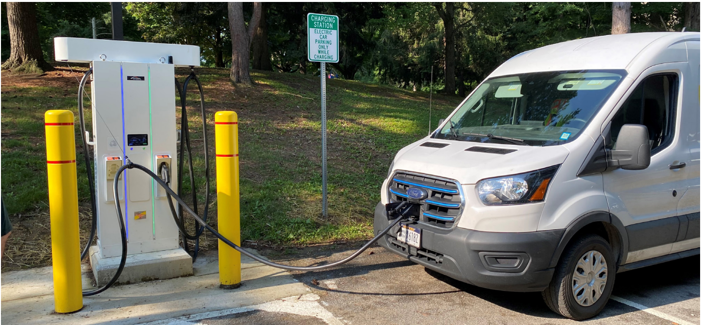
Level 3 EV Charger at Akron Falls Park
