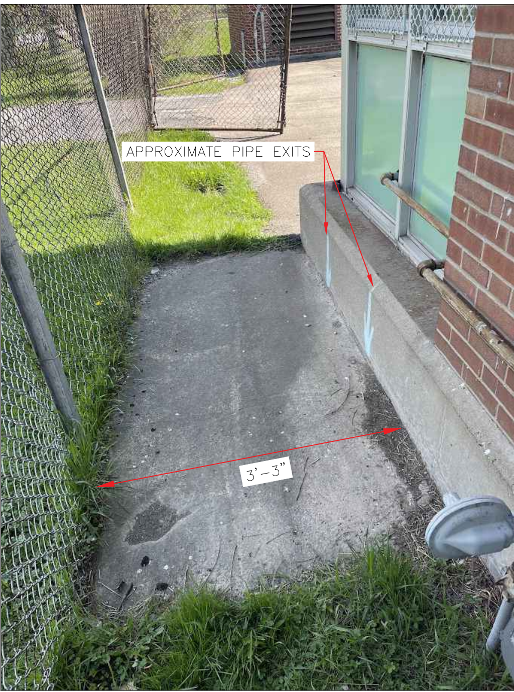
ROGERS ROAD PS FENCELINE
