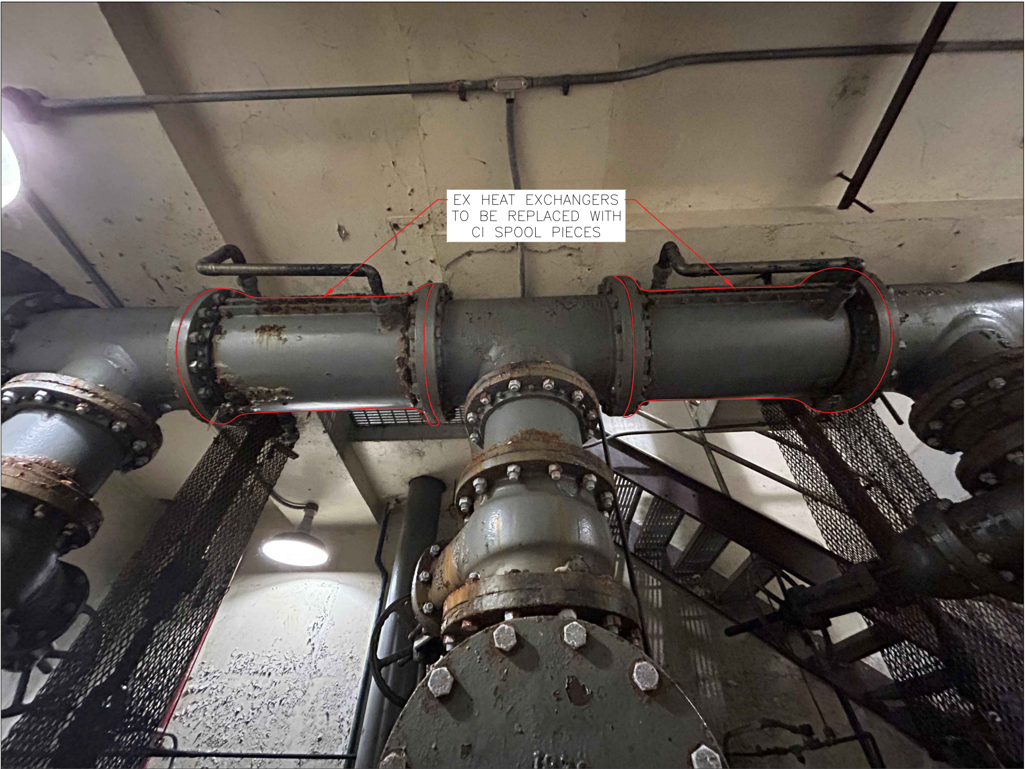
EXISTING PIPING WITH HEAT EXCHANGERS
